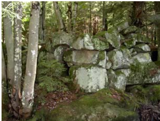
Photo 3: Remnants of the stone retaining wall
